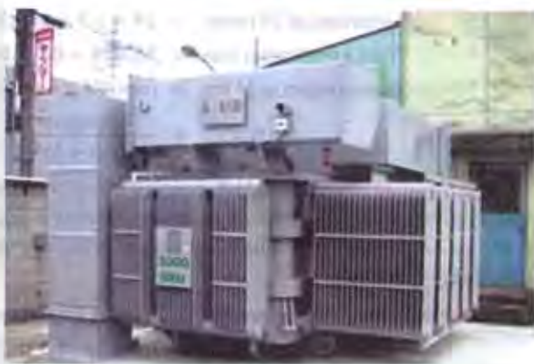
The world first 5,000 KVA amorphous transformer commissioned in August 2001 in Japan
