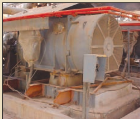
This 600 kW motor driving a refinery diesel pump suffered vibration and noise problems. After first dealing with soft footings, maintenance engineers eliminated resonance by adding bracing and new foundation bolts to the steel frame
