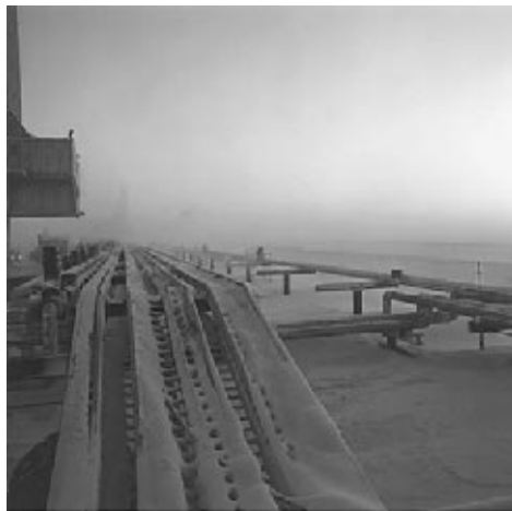
FIGURE 8 Field-based system installation at ARCO's West Sak field on Alaska's North Slope.
