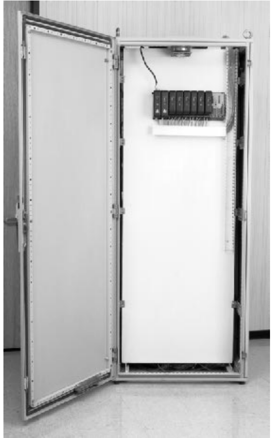
FIGURE 4 The nearly empty field-based system cabinet is shown with 384 I/O.
