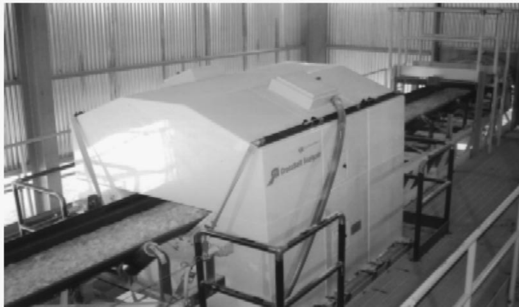
FIGURE 41 Cross-belt analyzer analyzing limestone rock on a 1000-mm trough belt at several hundred tonnes per hour.
