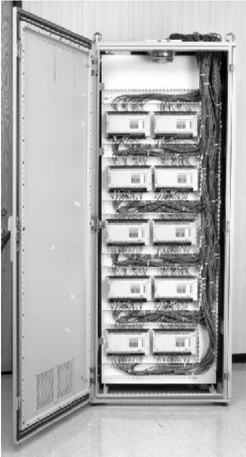
FIGURE 3 Footprint is significantly reduced when FOUNDATION fieldbus is used. The full cabinet handles 320 inputs and outputs (I/O).
