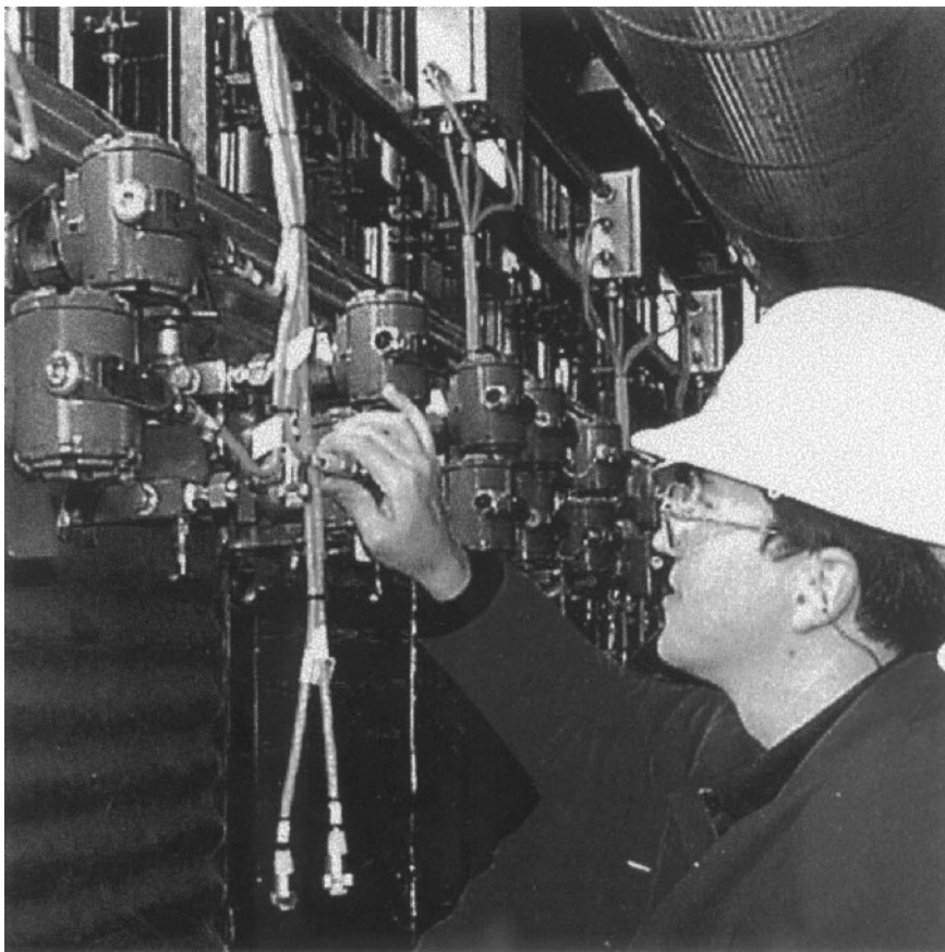
FIGURE 18 World's first large commercial installation based on the IEC/ISA fieldbus standard.
