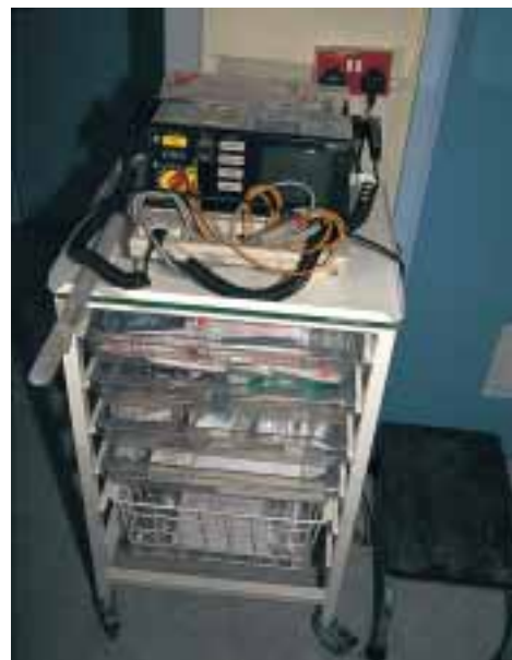
A defibrillation station should be prominent in areas of high risk
