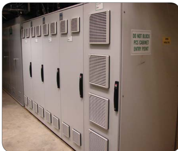
Figure 1. These new cabinets are located in the cable-spreading room in a mild environment that is air conditioned and heated to 66 °F.
