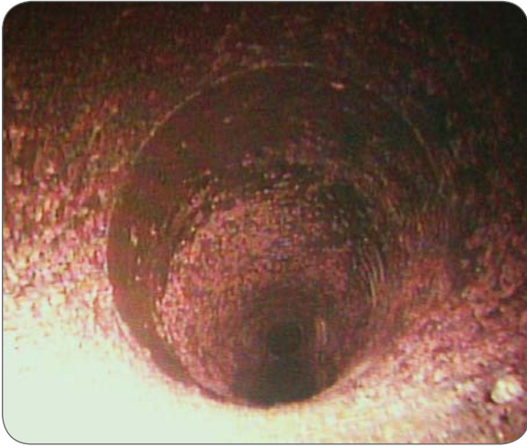
Figure 7. Swirl encrustation “fossilized” onto straight pipe wall.
