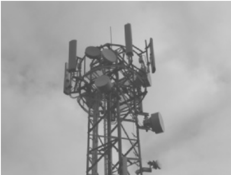
Figure 5.57 Installed antennas and supporting structure
