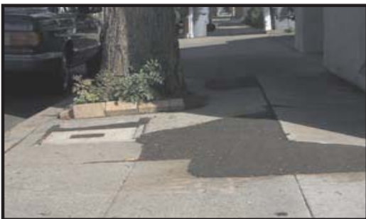
Severely damaged sidewalks such as this can be hazardous to pedestrians and costly to repair.
