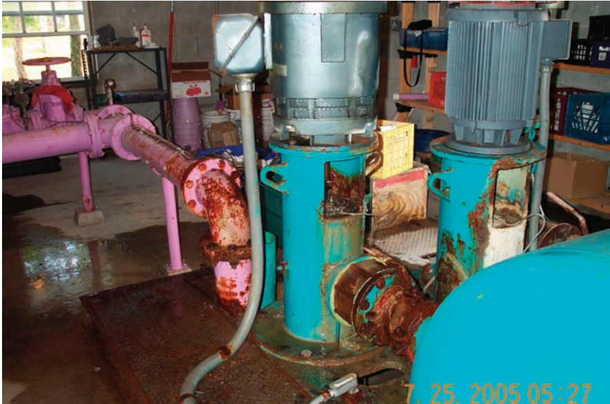
FIGURE 4 Accelerated corrosion by chlorine gas vapors resulting from recycled water being delivered directly into wet well of the pump station. Highly chlorinated recycled water should be delivered into open reservoirs to allow the corrosive vapors to release into the atmosphere (Tampa, FL).
