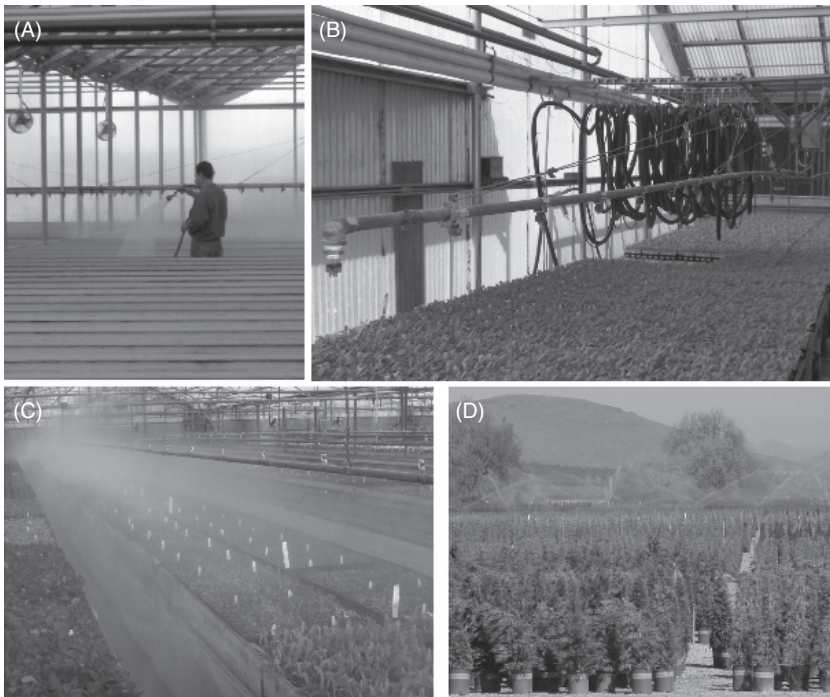
FIGURE 4.3 Overhead irrigation systems: (A) Hand watering, (B) Boom system, (C) Mist system, (D) Sprinkler system in an outdoor nursery (see also Plate 4).
