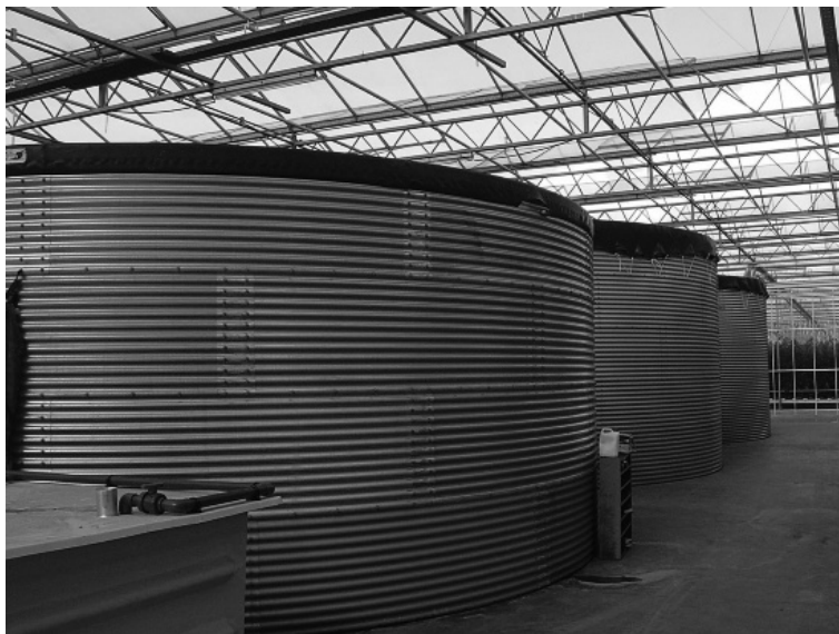
FIGURE 5.1 Rainwater storage in metal tanks (see also Plate 7).
