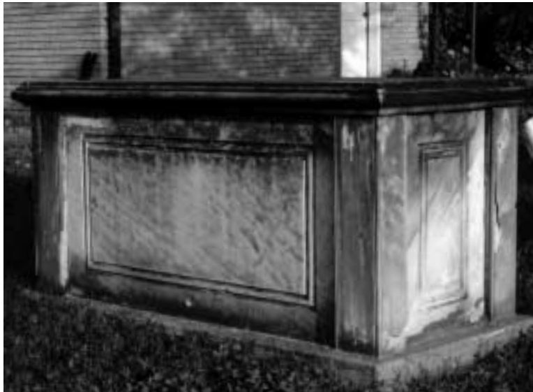
A box tomb in fairly good condition. Note the stone delaminating on the right corner of the monument.
