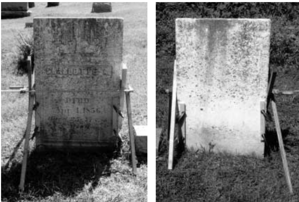
After the repair has been made, securing the marker is imperative. The use of clamps, wooden braces and shims assures the marker is not touched by the metal clamps, and also prevents the marker from moving while the repair treatment cures.
