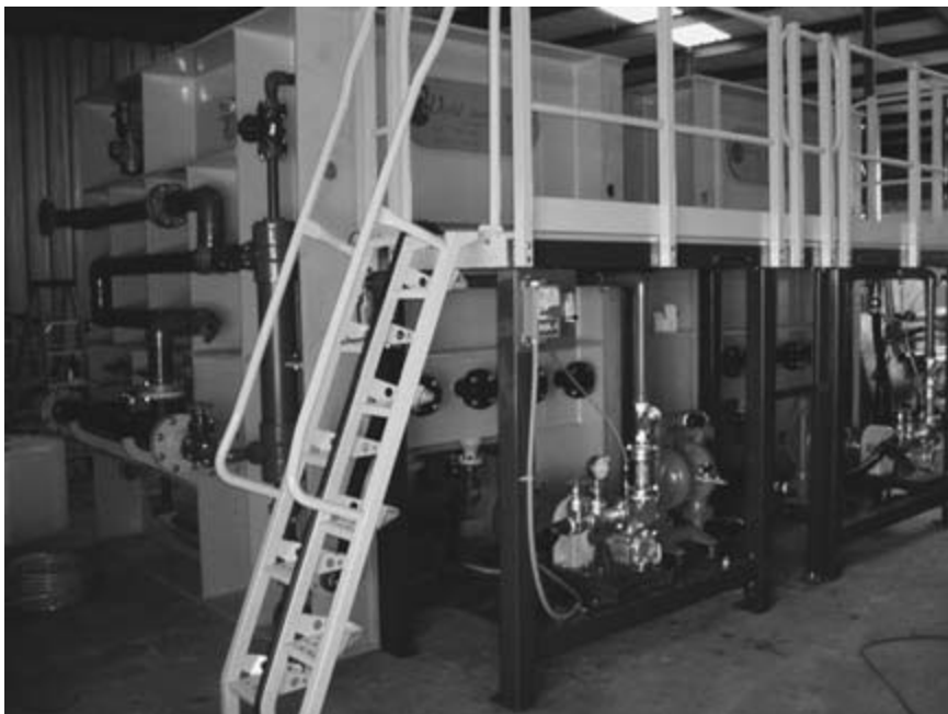
Figure 3.5. A photo of a dissolved air flotation system.
