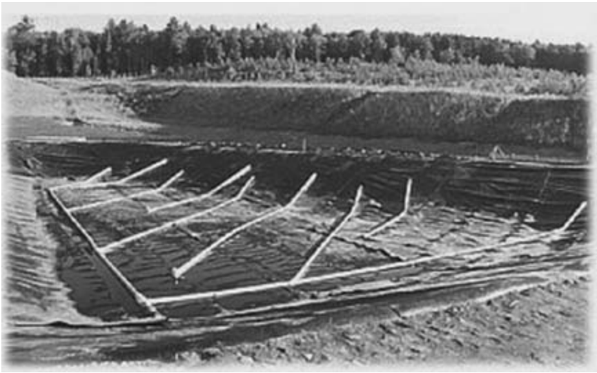
Figure 7.3. A photo of a reed bed sludge treatment before planting vegetation.
