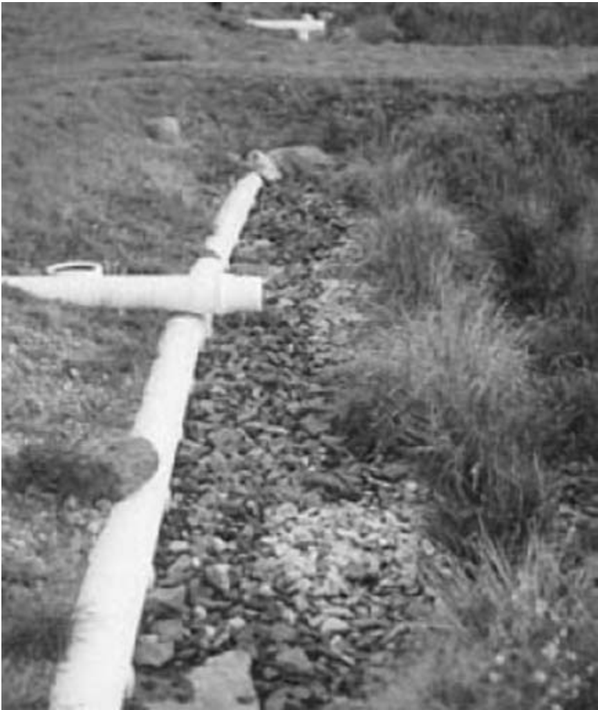
Figure 6.11. A subsurface flow wetland system in the U.S. (courtesy of USEPA).
