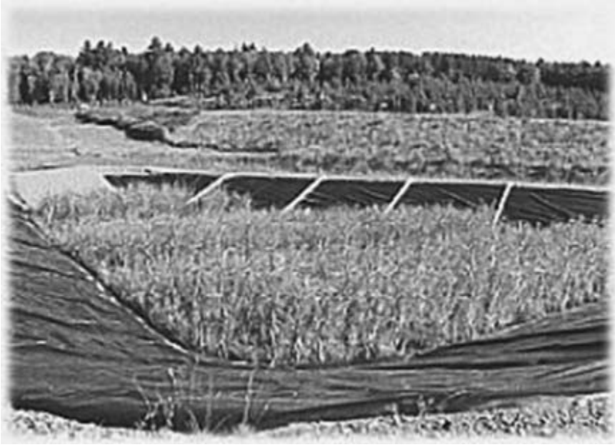
Figure 7.4. A photo of a reed bed sludge treatment after planting vegetation.
