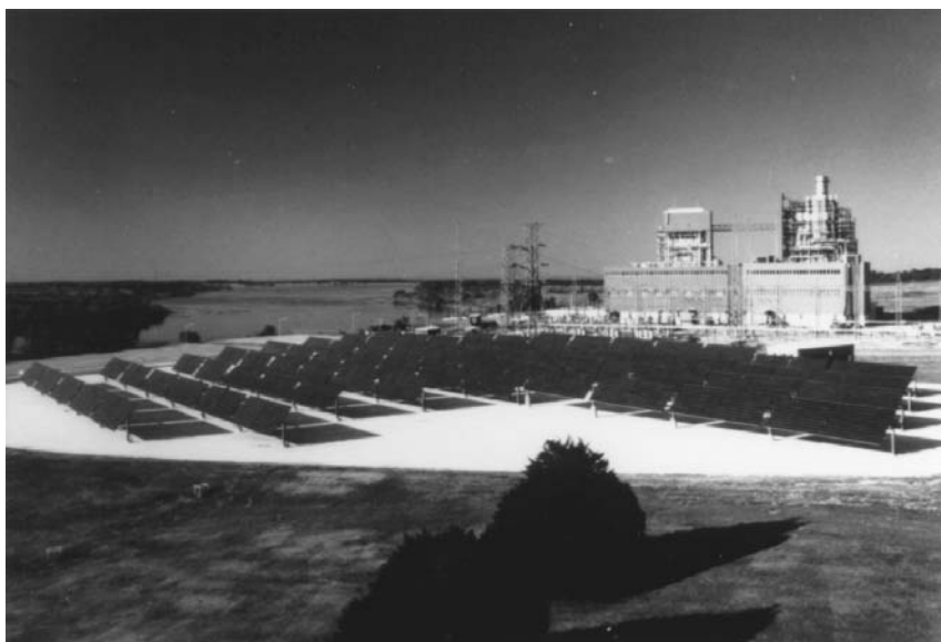
FIGURE 60.2 A view of the city of Austin PV-300 flat-plate grid-connected photovoltaic system. (Courtesy of the city of Austin electric utility department.)
