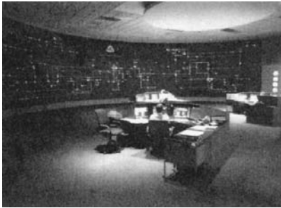
FIGURE 67.1 Central dispatch operation arena of Entergy Corporation's Beaumont Control Center (Beaumont, Texas) which includes a modern EMS.
