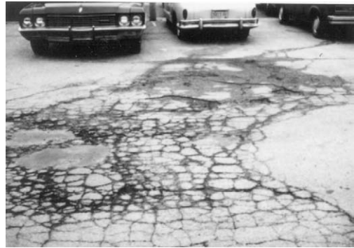
FIGURE 8.16 Alligator cracking developed due to cycles of freeze and thaw combined with poor drainage.
