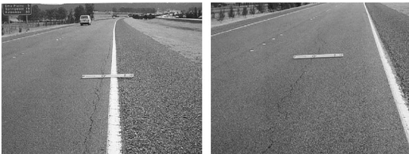
FIGURE 19.10 Longitudinal cracks in flexible pavements (Source: Austroads, 1987).
