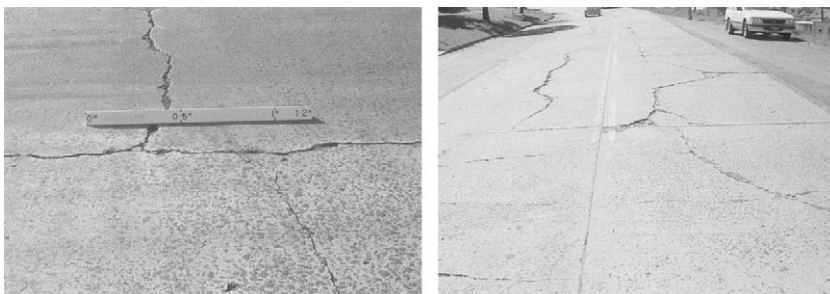
FIGURE 19.32 Block cracks in rigid pavements (Source: Austroads, 1987).
