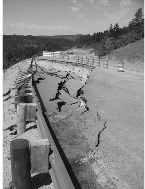
FIGURE 13.1 Catastrophic slope failure.
