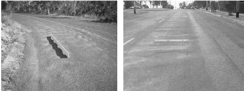
FIGURE 19.4 Corrugations in flexible pavements (Source: Austroads, 1987).
