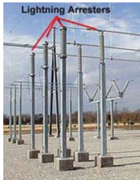
Lightning arresters on bus structures
