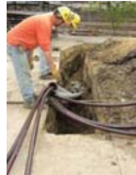
Underground transmission system.
