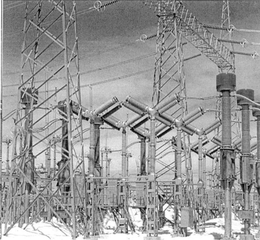
Fig. 6.70 AC breakers and current transformers at Radisson converter station, James Bay, Canada. Design temperature is -50^{\circ}\text{C} . (Courtesy of ABB, Sweden.)
