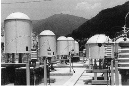
FIGURE 2.9.43 Installation of harmonic filter reactors for an HVDC project with a sound-shield enclosure.
