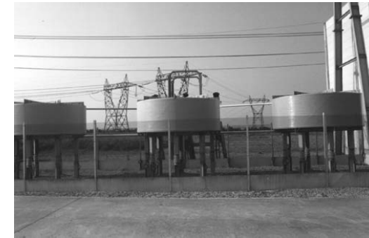
FIGURE 2.9.20 20-kV, 20-MVA (per phase) dry-type, air core, tertiary-connection shunt reactors.
