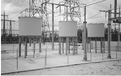
FIGURE 2.9.8 230-kV bus-tie reactors.
