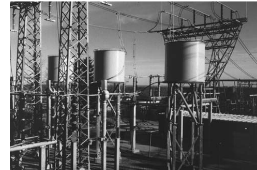
FIGURE 2.9.6 345-kV phase reactors.
