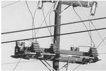
FIGURE 2.6.29 5-kV three-phase/four-wire metering rack with 3 VT and 3 CT. (Photo courtesy of Kuhlman Electric Corp.)
