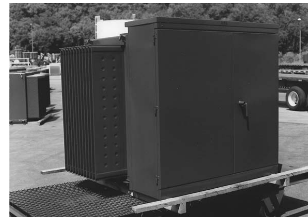
FIGURE 2.2.2 Typical three-phase pad-mounted distribution transformer. (By permission of ABB Inc., Jefferson City, MO.)
