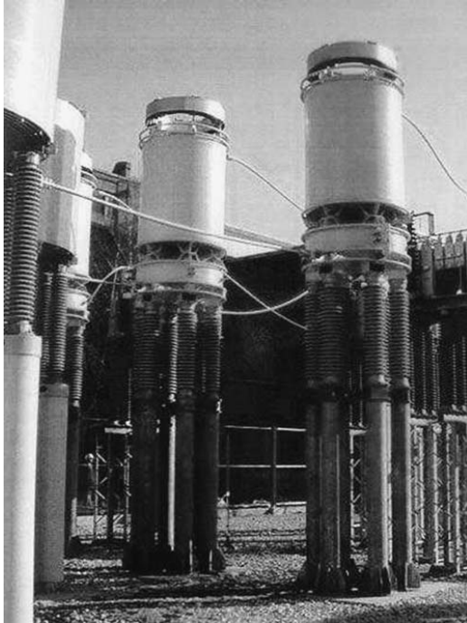
FIGURE 2.9.39 Tapped filter reactor with de-Q'ing rings.
