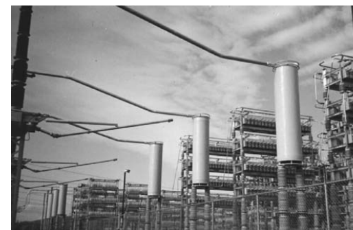
FIGURE 2.9.16 550-kV capacitor inrush/outrush reactors.
