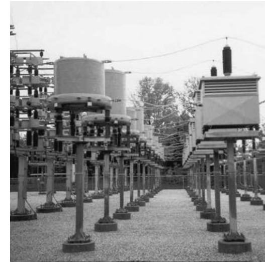
FIGURE 2.9.38 AC filter for an HVDC project; capacitors, tapped filter reactors, and separately mounted resistors.
