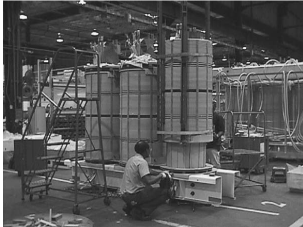
FIGURE 2.1.8 Concentric arrangement, outer coil being lowered onto core leg over top of inner coil.
