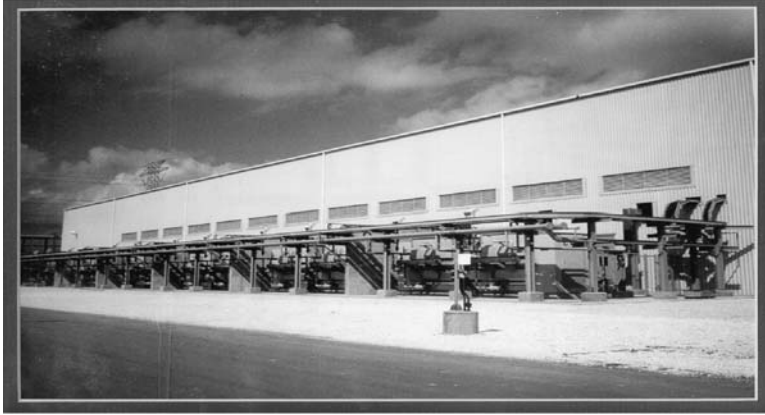
FIGURE 2.4.21 A 36-pulse system made up of 12 transformers with six types of six-pulse transformers for high-current electrochemical rectifier duty. Each transformer is 11,816-kVA OFWF with 426-V delta secondary windings. Each transformer has a 34,500-V primary with the shifts shown in Table 2.4.7 for a 36-pulse system. (Photo courtesy of Niagara Transformer Corp.)
