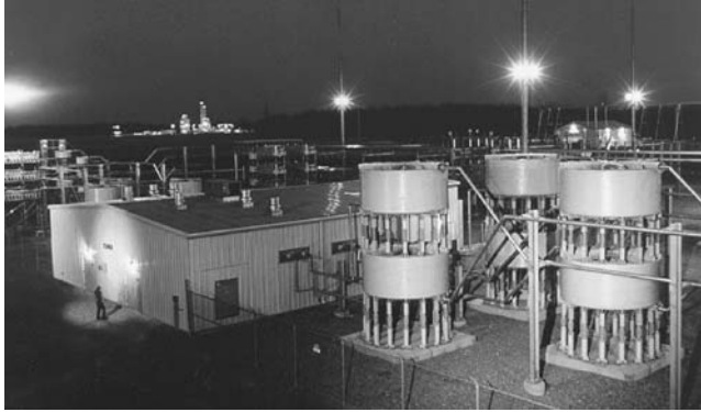
FIGURE 2.9.23 34-kV, 25-MVAR (per phase) thyristor-controlled reactors.
