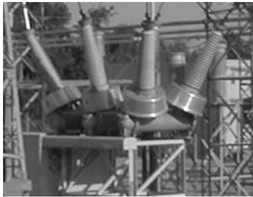
FIGURE 2.6.28 High-voltage circuit breaker with BCTs mounted underneath a metallic cover. (Photo courtesy of Kuhlman Electric Corp.)
