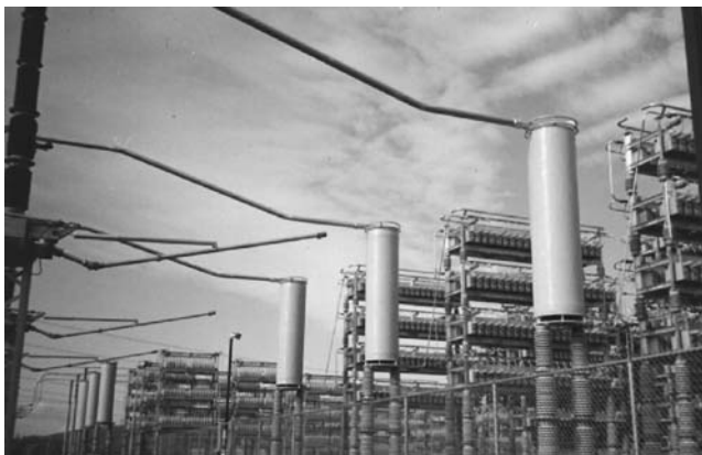
FIGURE 2.9.16 550-kV capacitor inrush/outrush reactors.
