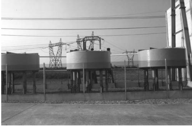
FIGURE 2.9.20 20-kV, 20-MVA (per phase) dry-type, air core, tertiary-connection shunt reactors.
