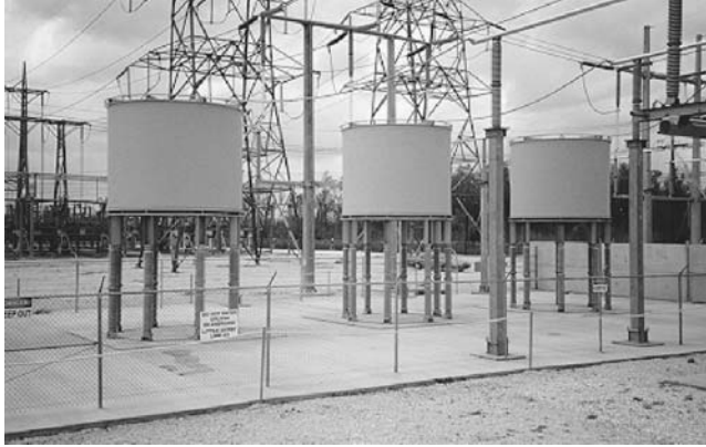
FIGURE 2.9.8 230-kV bus-tie reactors.
