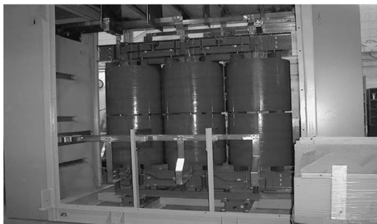
FIGURE 2.4.19 A 12-pulse Circuit 31 5450-kVA, 4160-V delta primary to 2080-V delta and wye secondaries, cast-coil transformer in case. (Photo courtesy of Niagara Transformer Corp.)
