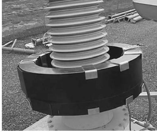
FIGURE 2.6.27 00-V-class slipover CT installed on high-voltage bushing with ground shield. Note the ground lead going back through the CT window to avoid shorted electrical turn. (Photo courtesy of Kuhlman Electric Corp.)
