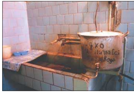
Ward kitchen sink in a Baku children's hospital
